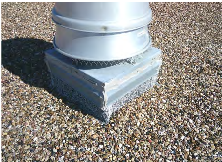
8. Asbestos Homogeneous Area 4 – Gray / white sealant on metal joints for roof equipment, vents, etc.; Sample 04
