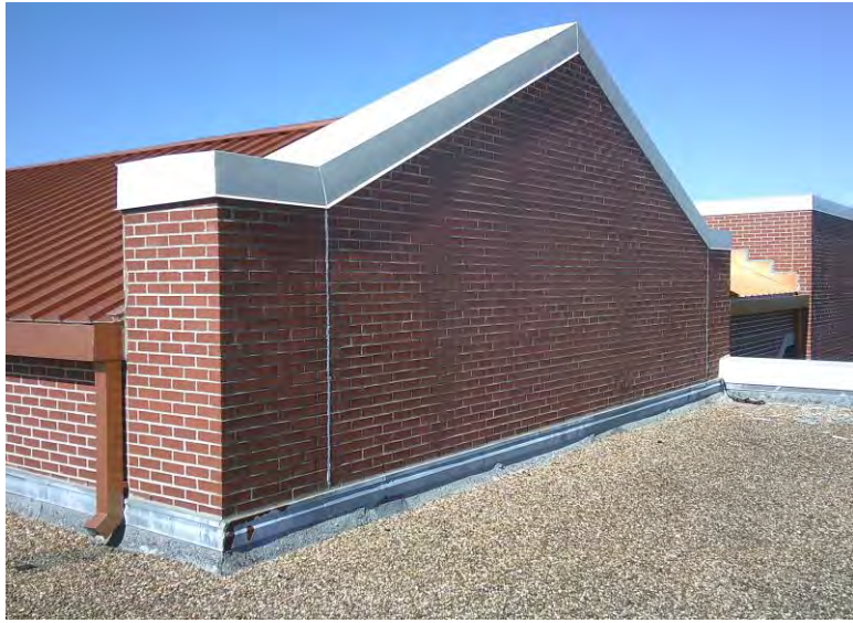
13. Asbestos Homogeneous Area 9 – Tan / white / gray vertical wall and flashing joints sealants; Sample 09
