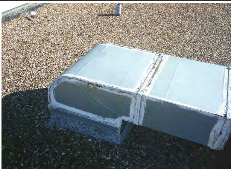
9. Asbestos Homogeneous Area 4 – White / gray sealant on metal joints for roof equipment, vents, etc.; Sample 04
