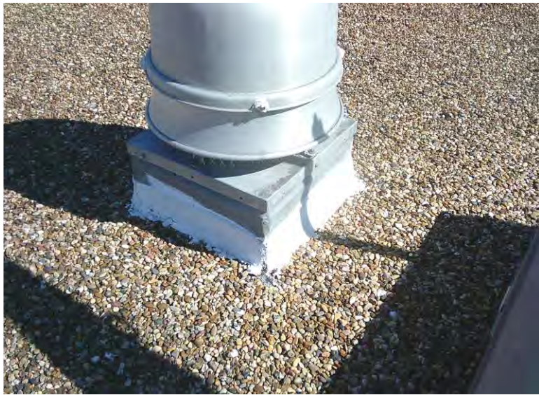
7. Asbestos Homogeneous Area 3 – White sealant on metal joints for roof equipment, vents, etc.; Sample 03
