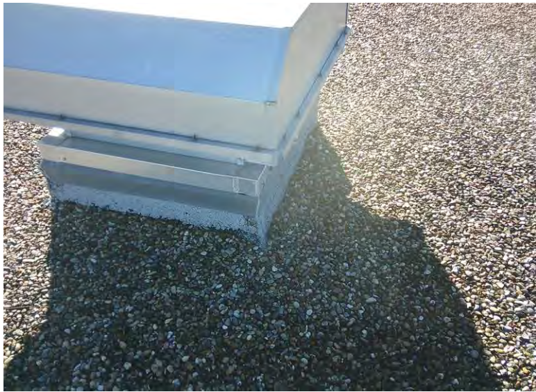
7. Another view of Asbestos Homogeneous Area 2 – Gray / black roof perimeter edge and penetrations flashing materials; Sample 02
