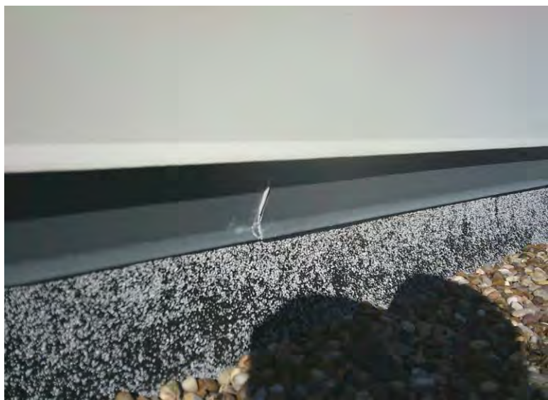
11. Asbestos Homogeneous Area 6 – White / gray metal flashing drip edge joint sealant; Sample 06
