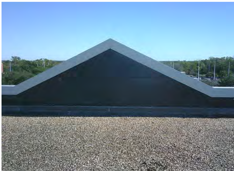
11. Asbestos Homogeneous Area 7 – Vertical wall rubber membrane and black / gray sealant materials; Sample 07
