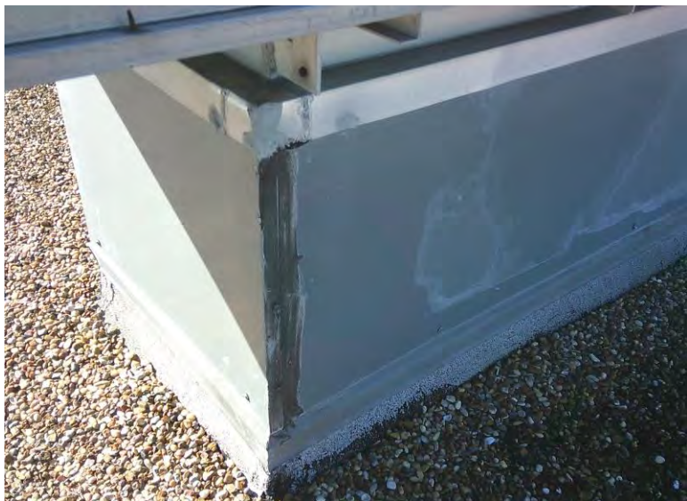
8. Asbestos Homogeneous Area 3 – Gray sealant on metal joints for roof equipment, vents, etc.; Sample 03
