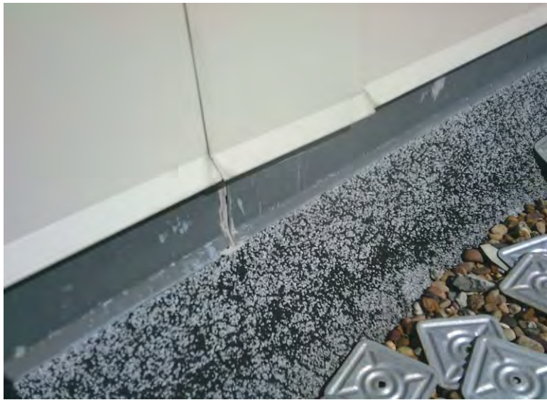
10. Asbestos Homogeneous Area 6 – White / gray metal flashing drip edge joint sealant; Sample 06
