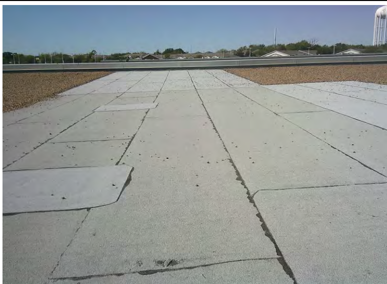
12. Asbestos Homogeneous Area 8 – Gray / black roll roofing materials and seam sealant; Sample 08
