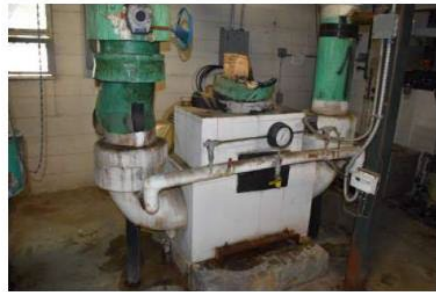
Existing Equipment: Outdated and Ready for Replacement
