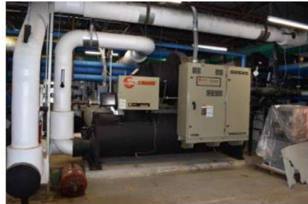
Existing Equipment: Re-use for Cost Savings
