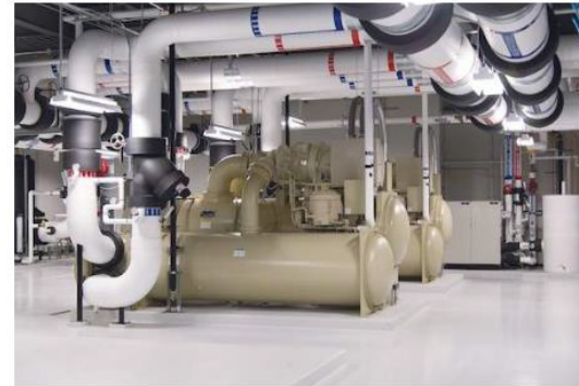
The future central plant will feature new, energy efficient equipment
