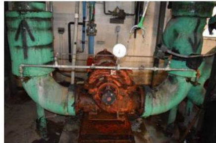
Existing Equipment: Outdated and Ready for Replacement
