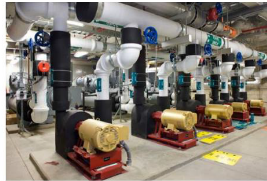
Example of pumps with common header
